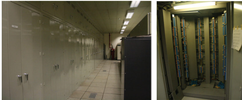
Fig. 1: I/O Cabinets and Wiring cabinet.
